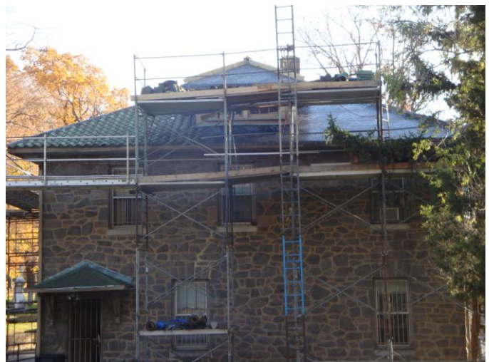
Tiles removed from north side gable roof and portion of the main roof; new underlayment installed
